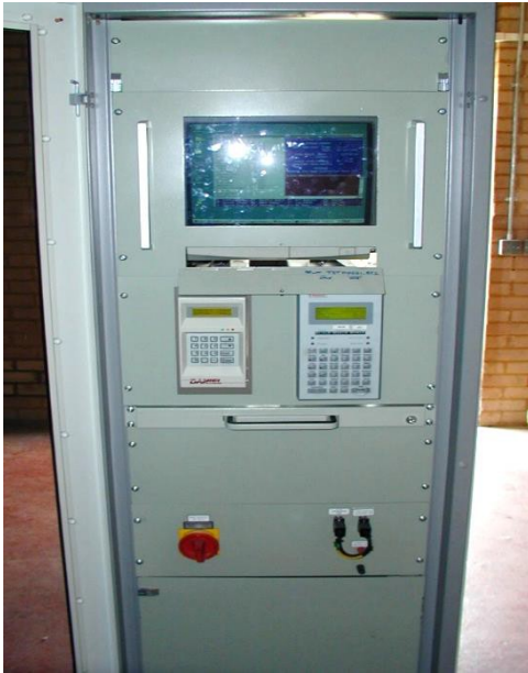
Figure 6: Current FWACV panel
