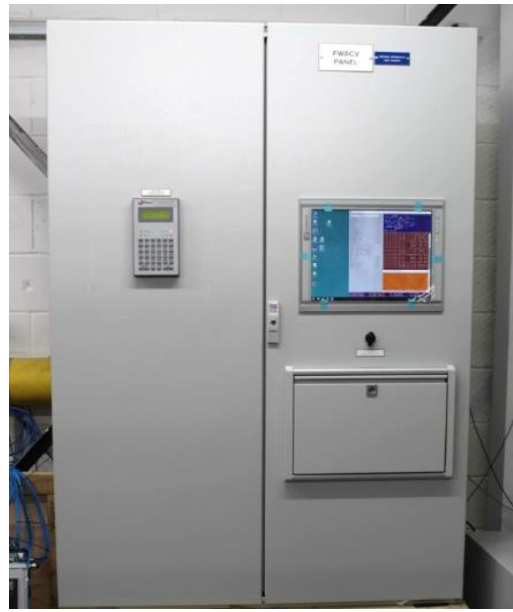
Figure 5: Modern FWACV panel
