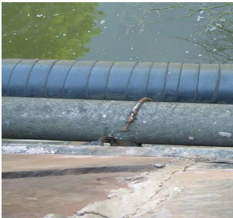
Figure 5: Failed clamp bracket, AC/PE main in the foreground, wrapped steel pipe at the back
