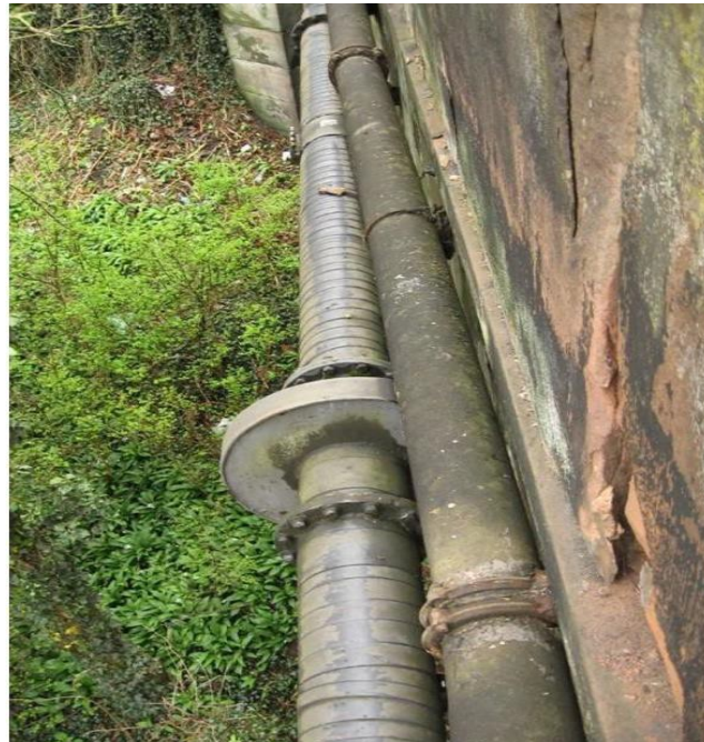
Figure 6: Unsupported AC/PE main resting on decommissioned steel pipeline
