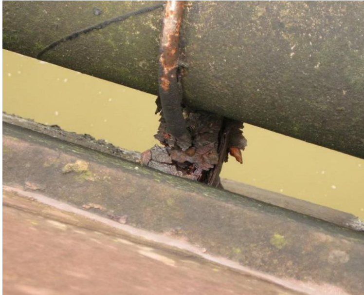
Figure 4: Example of deteriorating clamp bracket, the AC/PE main is at the top of the photograph
