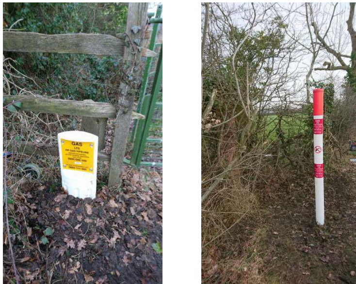
Figure 3 & 4: Upgraded CP test point for pipeline adjacent to sleeve together with marker post
