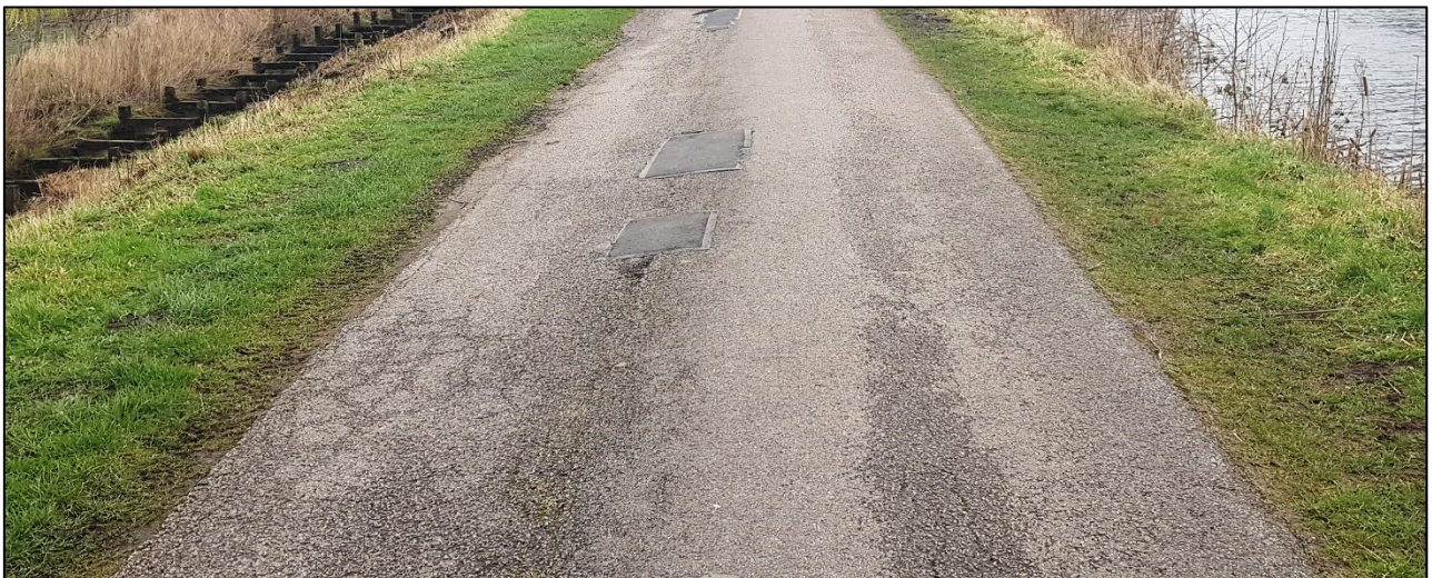
Figure 3-1 Examples of ongoing road rutting and damage from traffic
